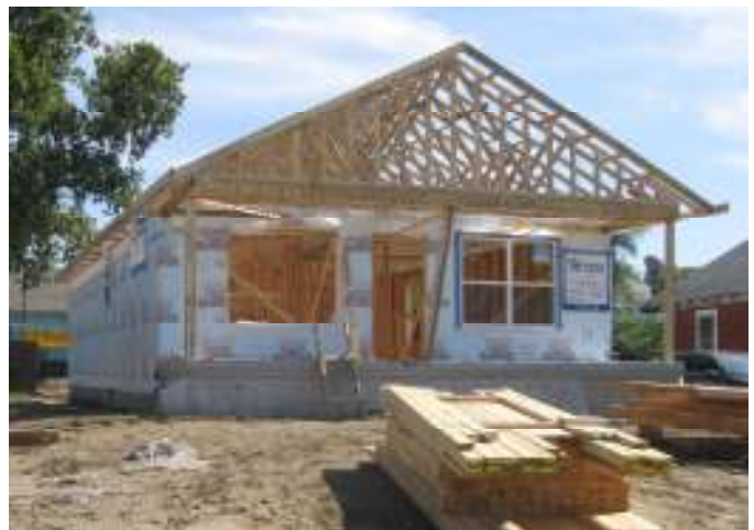
The roof trusses are in place, and some of the framing has begun on the inside of the house. (Photo taken on September 18)
